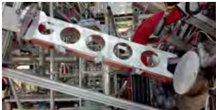
Fig. 1: Photograph of the optical remote-steering antenna (ORSA) during installation in W7-X.
